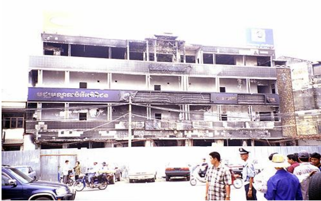
The offices of Cambodia Shinawatra Telecommunications, firebombed, windows smashed, with masonry damage.
